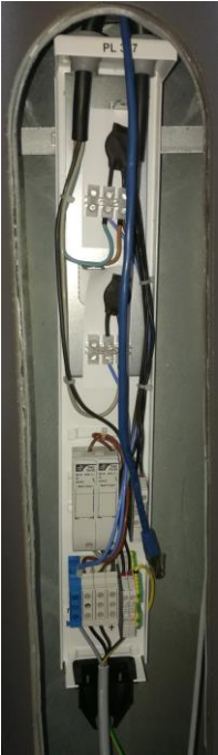
Figure 9 Trappe de raccordement
